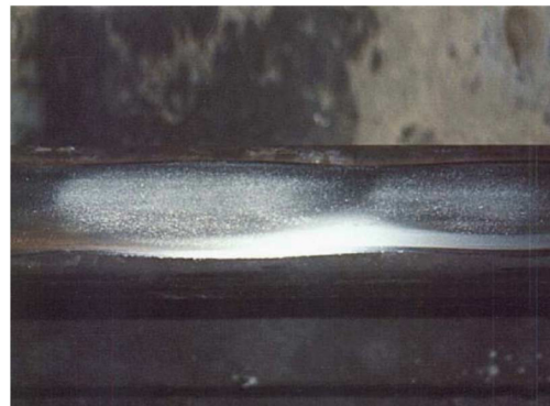
Fig. 7. Severe corrugation on the low rail of curve in a metro system.
