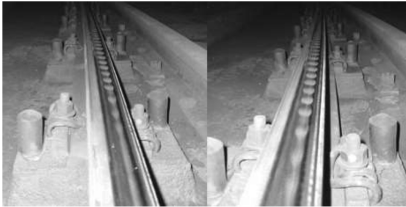
Corrugation development in curved track on a European metro system under dry conditions, 65 days after grinding
