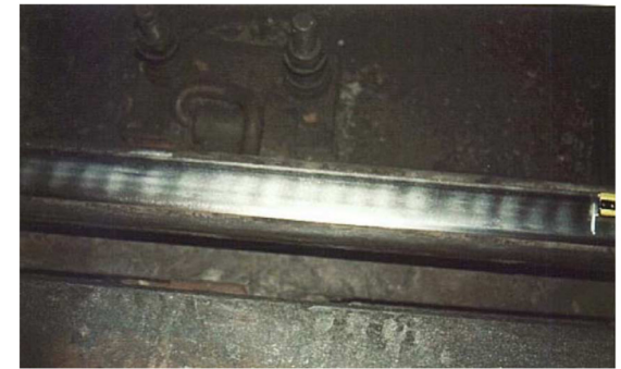
Fig. 8. Corrugation at 25–30 mm wavelength arising from excitation of the baseplate on the railpad.
